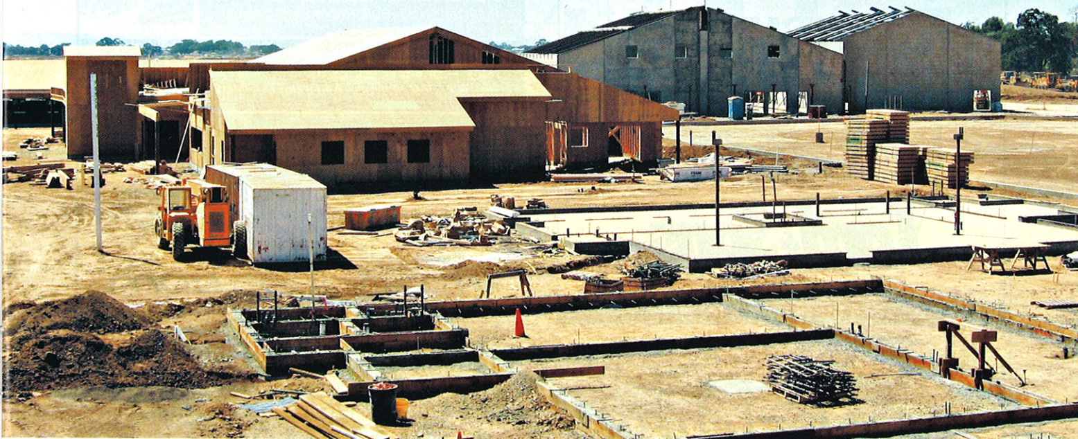
Construction crews work on one of the 27 buildings planned for the campus (photos courtesy of Lathrop Construction).
